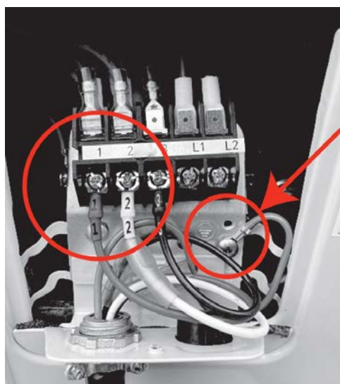
Ground wire Connection
